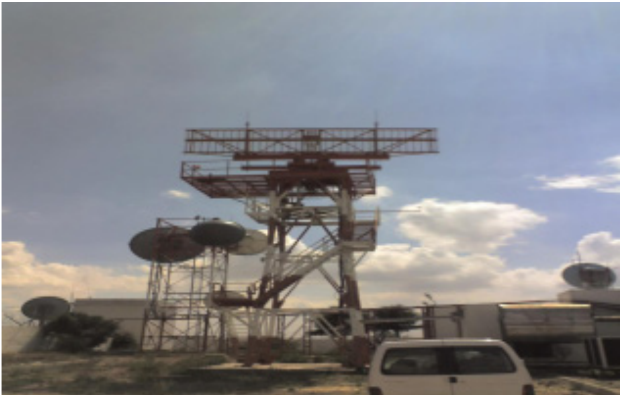
Figure 1: Station Radar Sidi Zid
